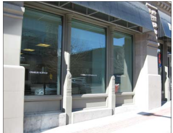
Cast iron columns embellish the window frame on the Brooks Arcade at 268 S. State Street.
