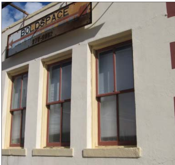
The number and position of glass panes in a window are important character-defining features of a building.
