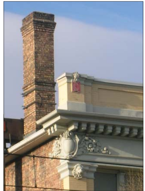
Chimneys can be an integral part of the roof composition.
