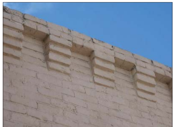
Salt Lake City commercial buildings offer a wide variety of cornice styles and materials, each helping to create the distinct character and identity of the building.
