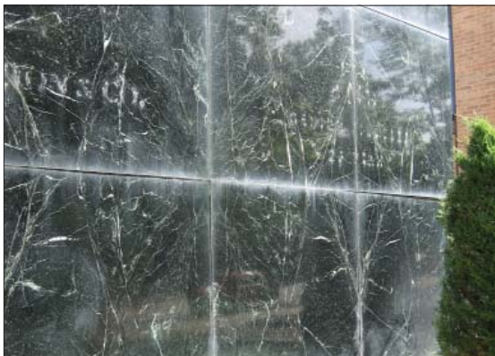
Marble paneled veneer on the main facade at 641-645 E. South Temple Street.
